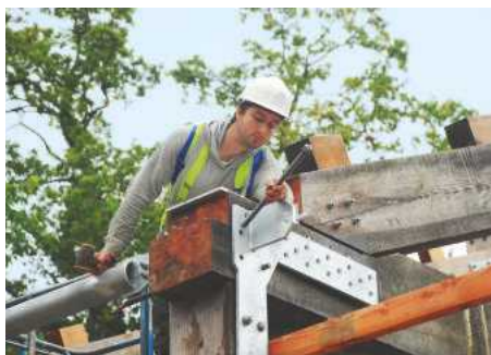
One of the four timber framers bolting a roof truss to its supporting timber
